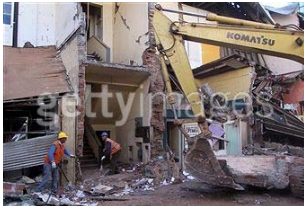
Damage caused by the earthquake.
